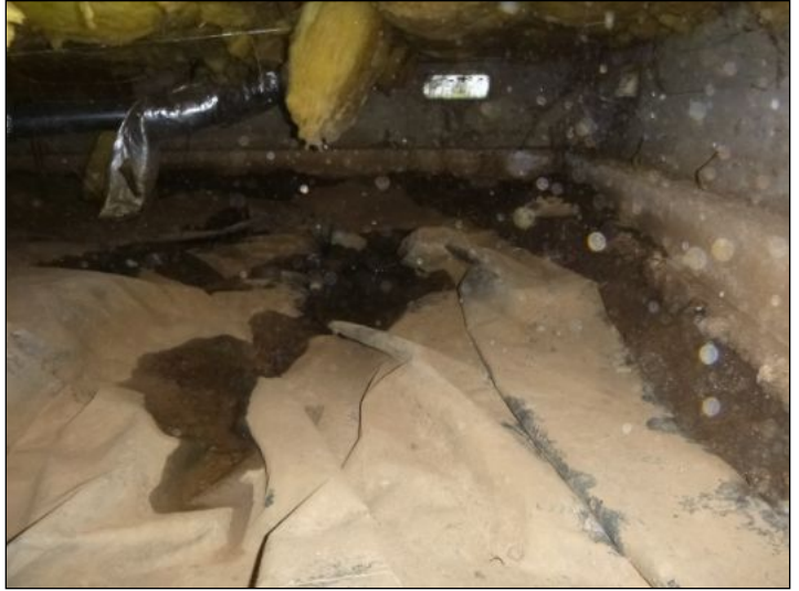
Pooling water in crawlspace.
