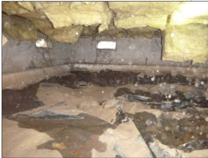
Pooling water in crawlspace. Displaced vapor barrier.
